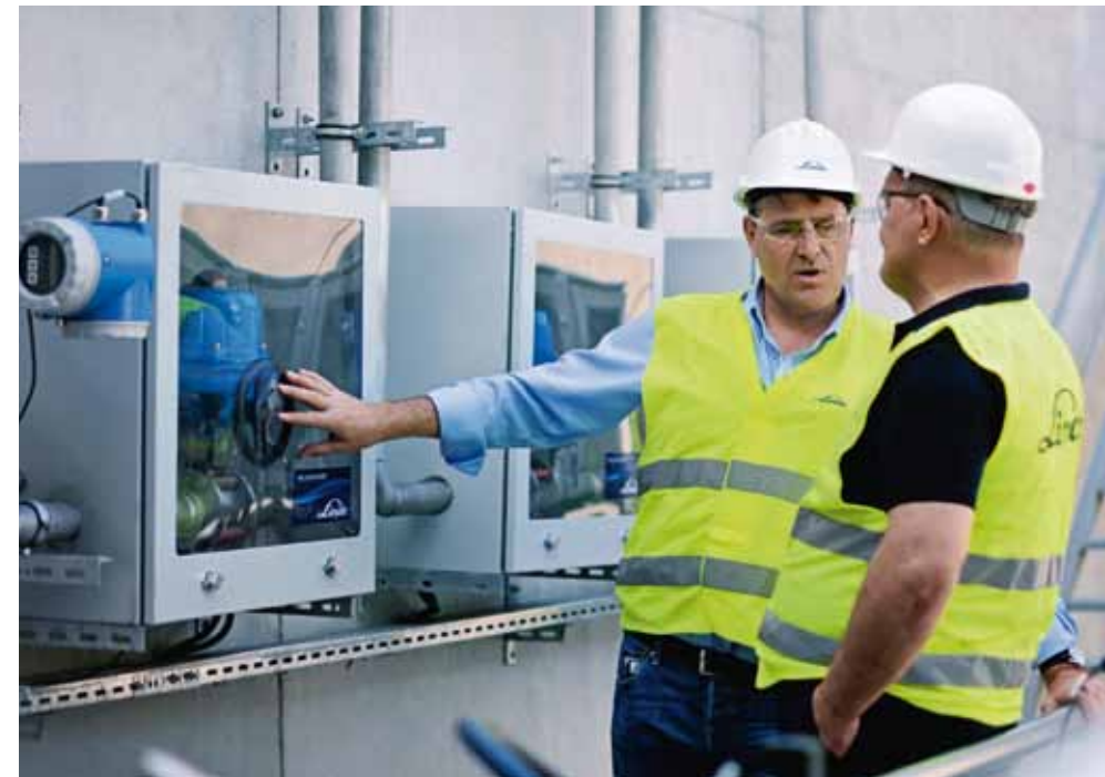
Darren Gurney, Senior Process & Business Development Manager (left), and Omer Saray, Applications Engineer (right), go over the details of the CO 2 dosing system.
